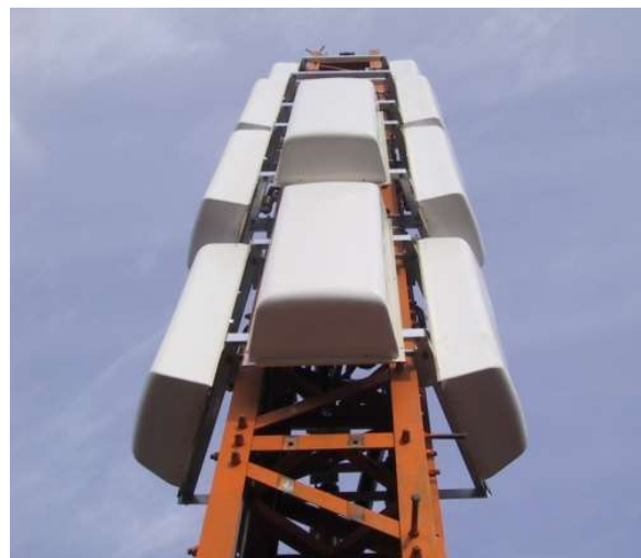
UHF DTV Antenna System in Gwang-gyo Site
